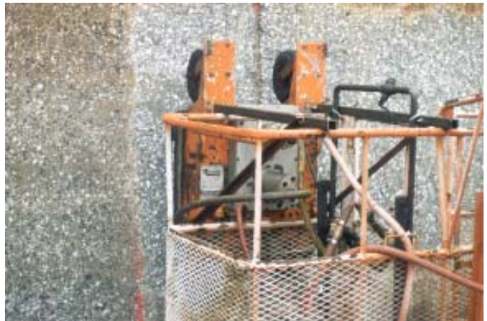
The NLB 20K SPIN JET is moved along the wall with a man lift, allowing for quick and efficient application of the high-pressure water.
