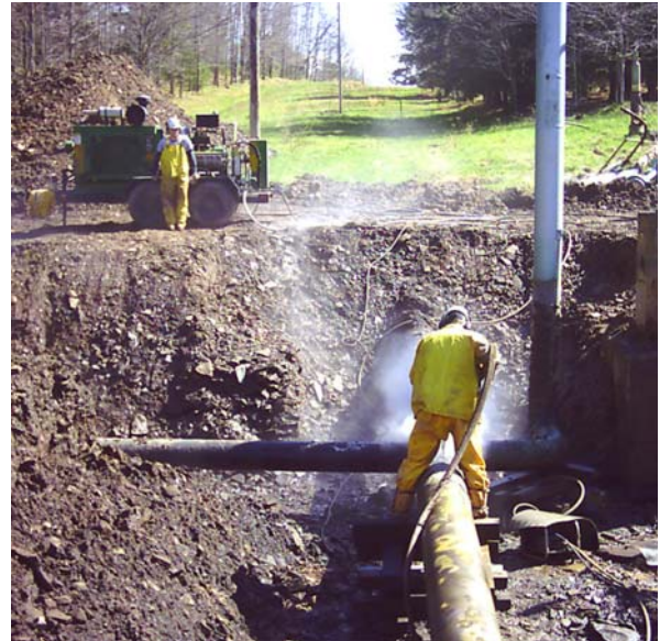
With two operators, the pipe coatings were removed in only one day.
