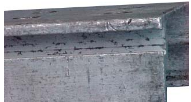
The "keyway" on the piece of staging with all concrete residue removed.
