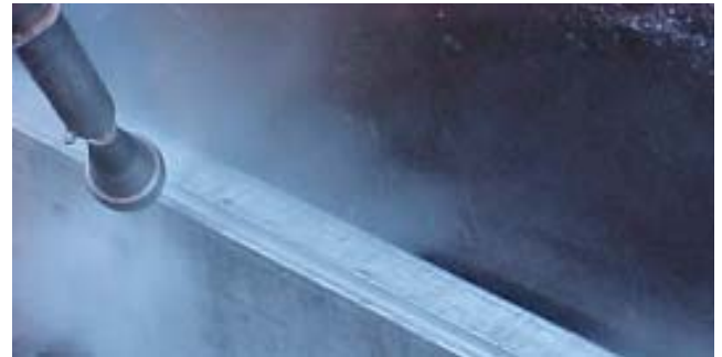
An NLB8400A-2 rotating lance cleaning out the concrete using ultra-high pressure water.
