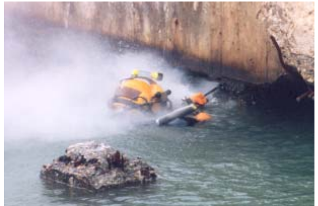
A diver working at low tide performs clean-up after a beam has been removed. One of the columns that was reused can be seen in the foreground.
